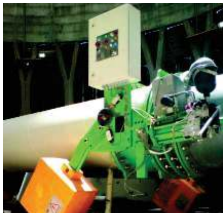
Normally close (fail to open) emergency Quick Discharge valve DN1800, PN10 DAMAVAND power plant, IRAN
